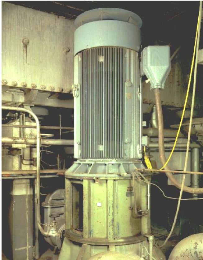
Pump drive, 800 kW, 6 kV 1493 rpm
