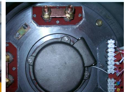
Main and auxiliary terminal box
